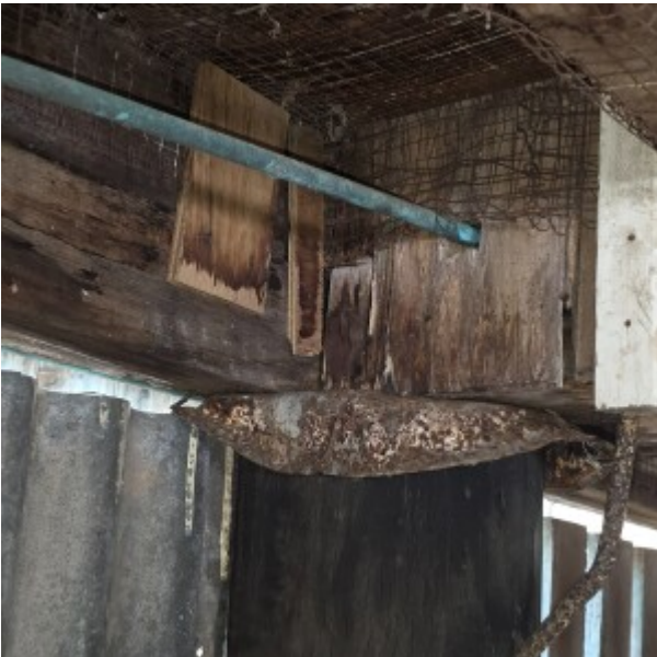
Rusted termite shield
