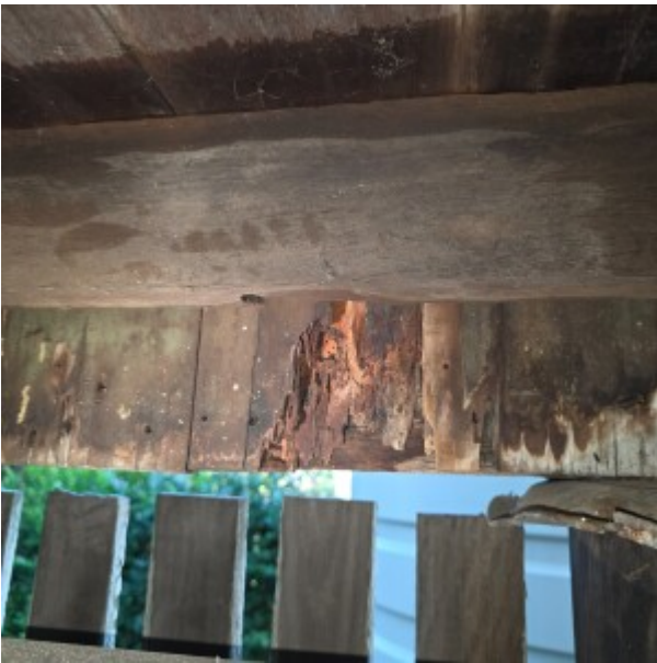
Damage in wall boards
