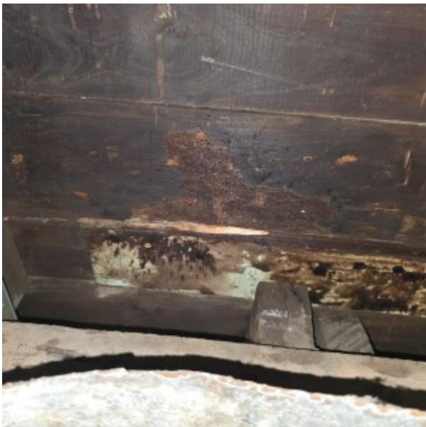
Damage in flooring
