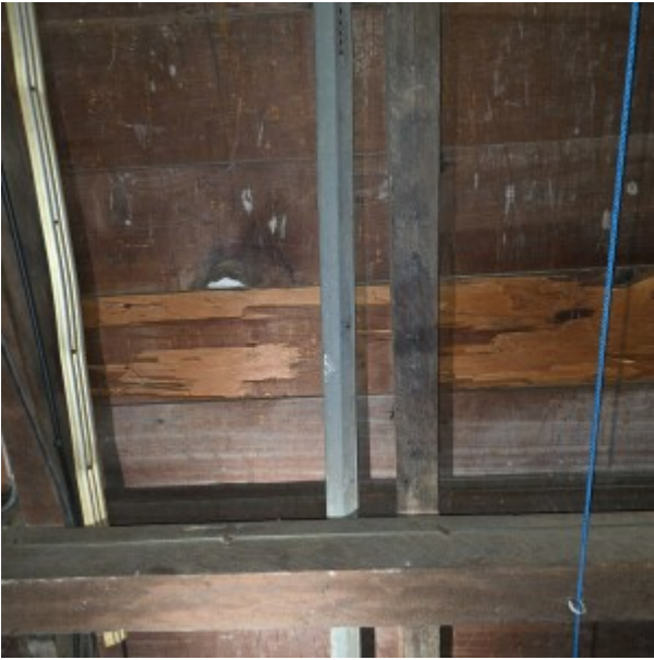
Damage in flooring
