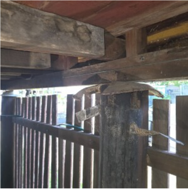
Damaged termite shields
