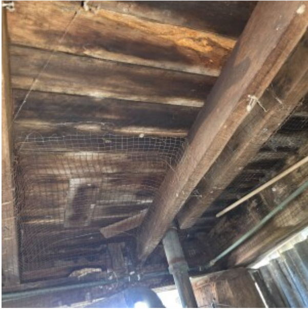
Damage in flooring
